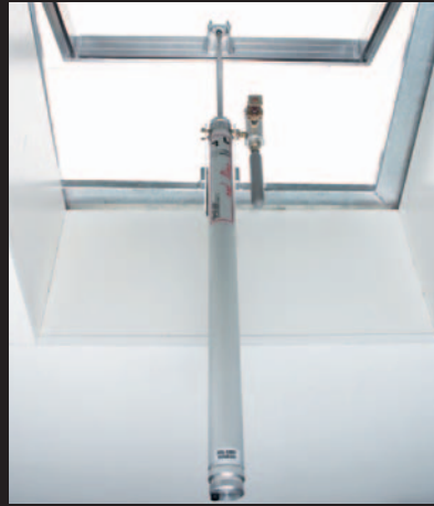
On dome with thermal valve
